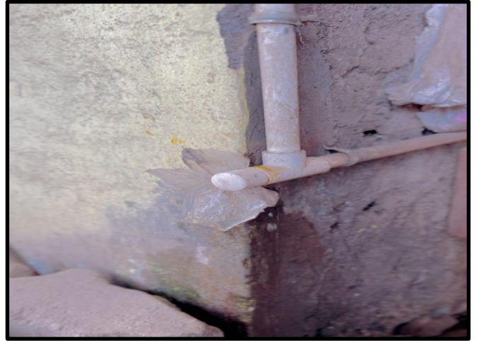
Water leakage in the locality
